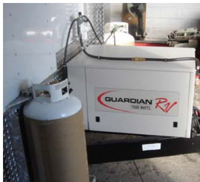
Propane Fueled Generator
